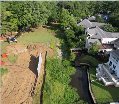
Retaining Wall Under Construction. Section Farthest From Camera Represents Most Closely the Final Height of the Wall.
